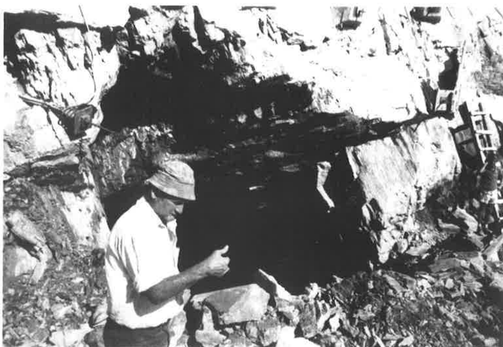
Fig 5. Genomslag. Lera och talk i sprickorna orsakar bergutfall trots förstärkningar. (Break Through. Clay and talk in joints causes overbreak inspite of heavy reinforcements)
