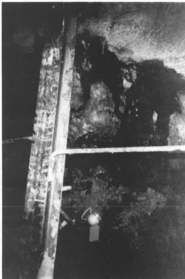
Fig 4. Jordomvandlat berg orsakar 2m utfall (Completely wheathered rock causes 2m overbreak)
