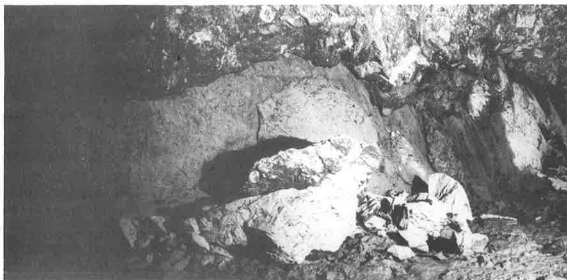
Figure 13 Right wall, Chainage 111. Rockfall of about 2 m 3 , including a 1.5 m 3 -sized block. This rockfall can be related to the steeply northward dipping joint. These blocks were also observed in 1971 (L. Runesjö, Håverud, oral comm. 1988).
