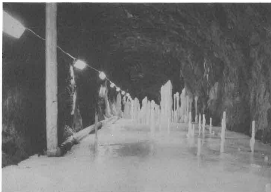
FIGUR 6 Delvis kalcitläkta sprickor i betongsprutat tunneltak Partly calcite-healed cracks in shotcreted roof of tunnel
